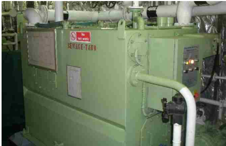
Sewage holding tank
